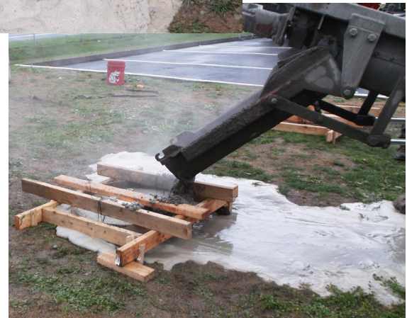
Water that accumulated in the two holes is displaced by the concrete.
