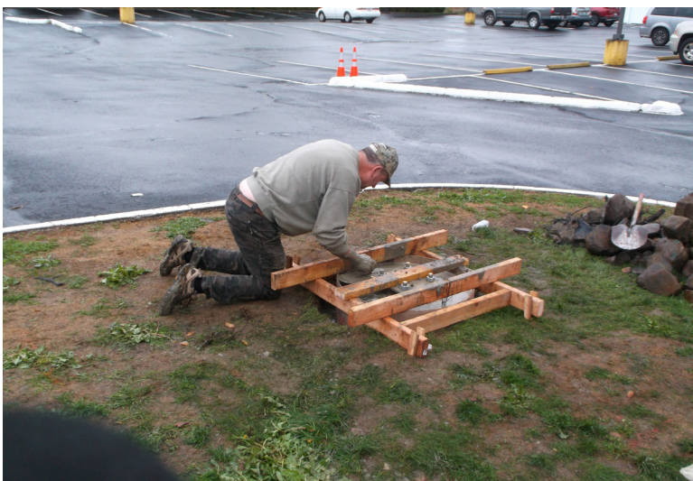
The last step in this process is to finish (smooth out) the surface of the newly poured concrete and clean-up the mess.
